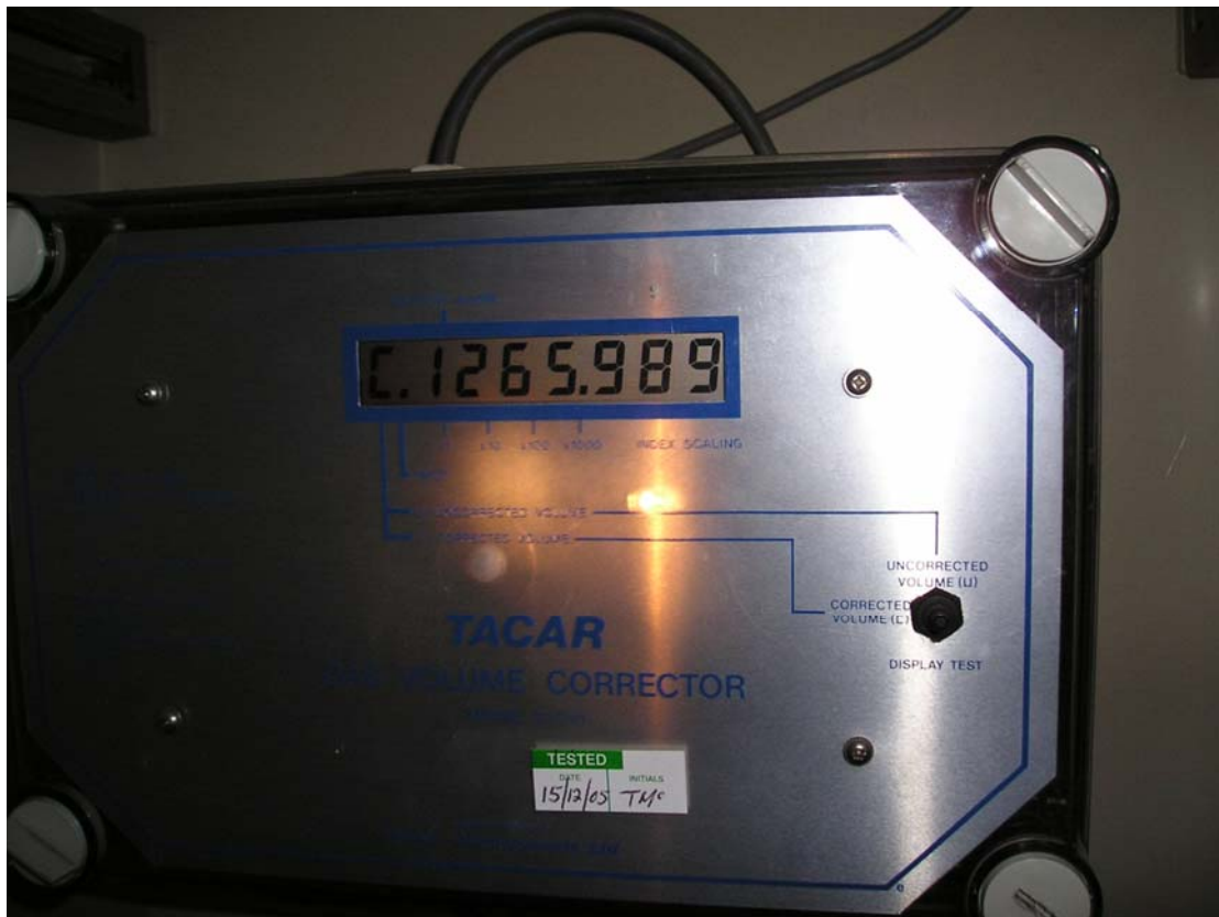
Figure 1: The interface of the gas corrector meter in the input pipe to Edinburgh University's central area combined heat and power plant. Photograph courtesy David Somervell, Estates and Buildings, University of Edinburgh.
